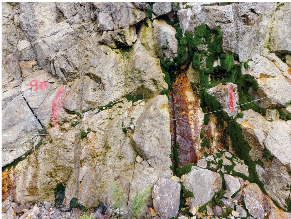
Figure 3. Scanline method: slope demarcation every 10 meters and investigation of slope conditions and structural measures.
