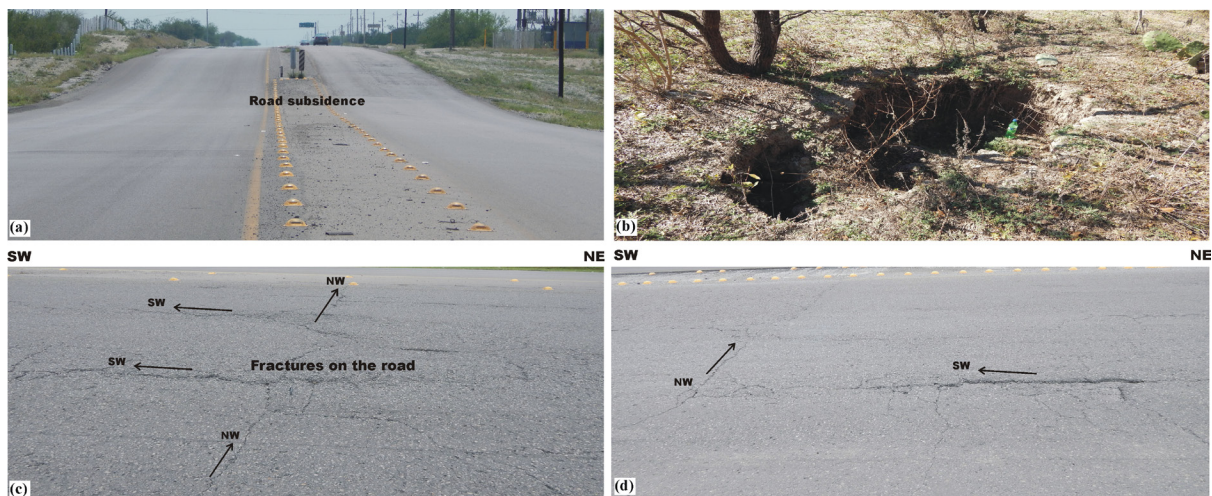
Figure 14. Sector 3. a) Image showing the subsidence of the road. b) Image of a sinkhole next to the road. c) and d) Images of fractures on the road surface in Profile P1. Reference points for the photographs shown in c) and d) are indicated as F1 and F2 in Figure 7, respectively.
