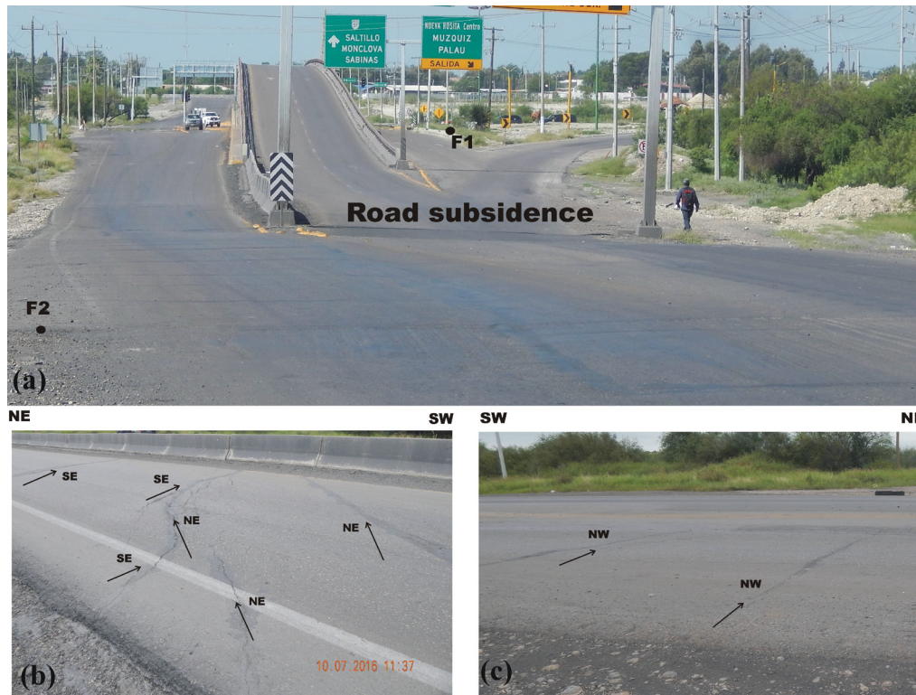
Figure 9. Sector 1. a) Image showing the subsidence of the road. b) and c) Image showing fractures on the road surface in profile P2. Arrows indicate location and direction of the fractures. Reference points for the photographs shown in b) and c) are indicated as F1 and F2 in Figure 2, respectively. F1 and F2 also are indicated in Figure 9a.
