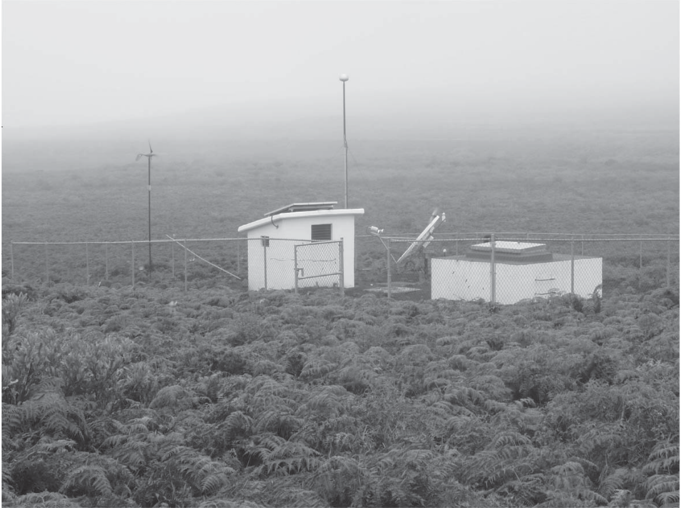
Fig. 2. Picture of station SRAD (H06E1) located near the landing strip and a now destroyed radar station. This is the eastern station of the network. The wind generator, the shed housing electric equipment with a solar panel on top, the lightning protection system, the satellite dish antenna and the seismic vault are shown.
