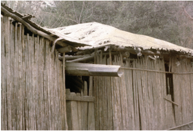
Fig. 6. Weak constructions damaged by ash fall and ballistic impacts (photo by S. De la Cruz-Reyna).
