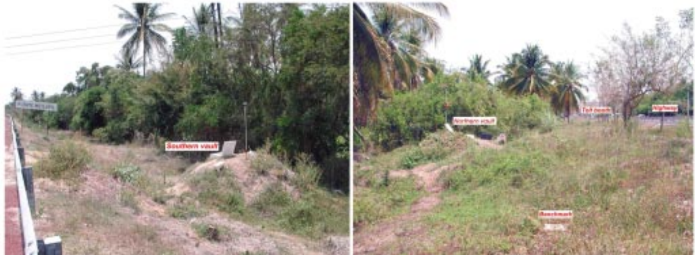
Fig. 10. LBT after installation. Left, southern vault. Right, northern vault with a benchmark in foreground and the highway tollbooth in the background. The vaults and the pipe are covered with at least 1 m topsoil to reduce temperature variation.
