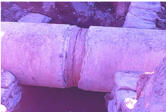
Fig. 4. Joint failure of a concrete pipeline after Mexico City earthquake, 1985.
