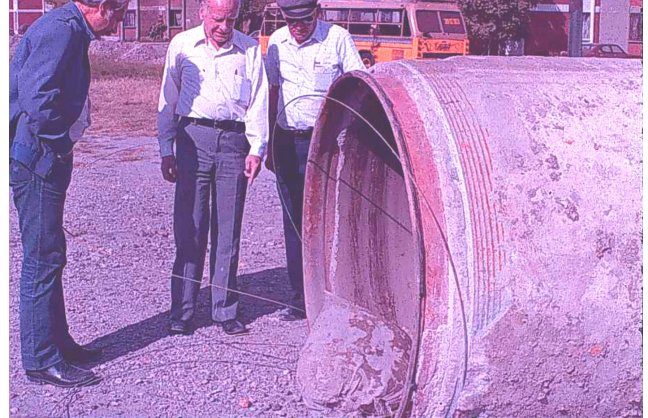
Fig. 5. Close view of a joint failure; Mexico City earthquake, 1985.
