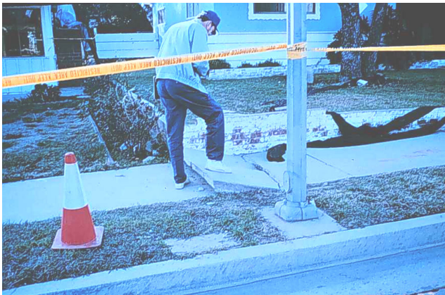
Fig. 3. Slab displacement due to permanent ground displacement. San Fernando valley, Calif. 1994 (Balboa Blvd).
