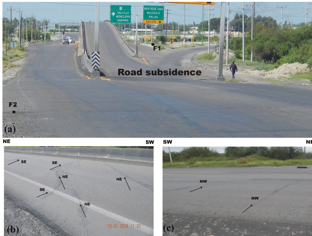
Figure 9. Sector 1. a) Image showing the subsidence of the road. b) and c) Image showing fractures on the road surface in profile P2. Arrows indicate location and direction of the fractures. Reference points for the photographs shown in b) and c) are indicated as F1 and F2 in Figure 2, respectively. F1 and F2 also are indicated in Figure 9a.
